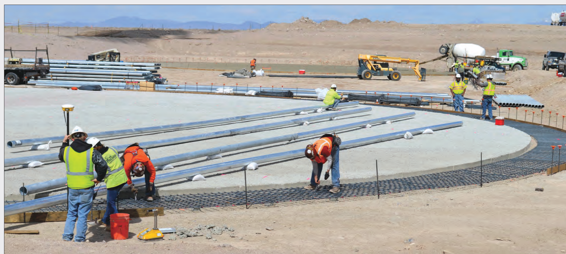
Hot prospect: pipes for cooling salt that has been heated by an array of mirrors being installed at SolarReserve's power generation project at Crescent Dunes, Nevada
