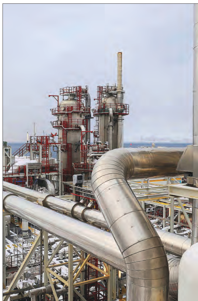
Pipe work: Statoil's gas processing plant near Hammerfest
