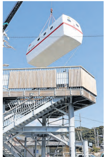
Floating shelter being installed on the top of a tsunami evacuation tower
