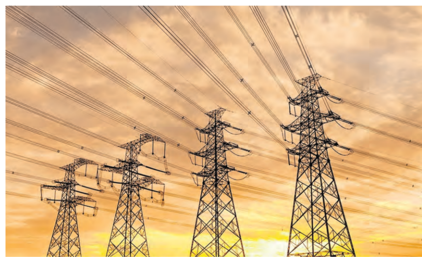
High tension: risks to technology that controls infrastructure grow – Dreamstime
