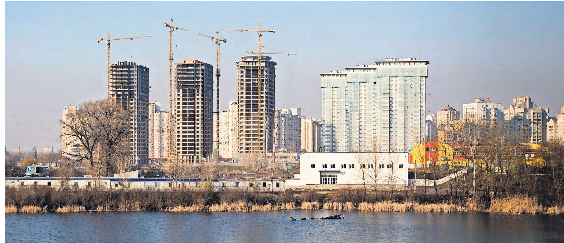
Life goes on: apartment blocks being built near the Dnieper river in Kiev, Ukraine
